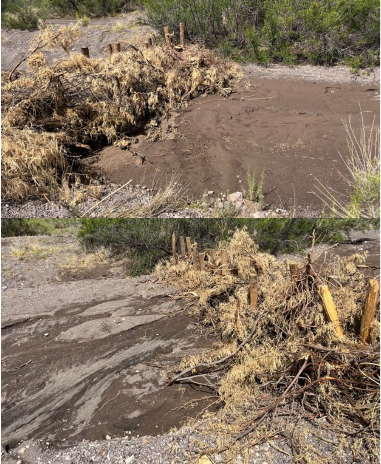
Figure 52. Brush weirs structures show uniformly-moist soil evidence of pooling, on the upstream side of structure (top) and more unevenly-moist soil on downstream side (bottom) after water has filtered through the structure after a mid-May 2023 flow event in creek. (Photo by Philip Boyd)
