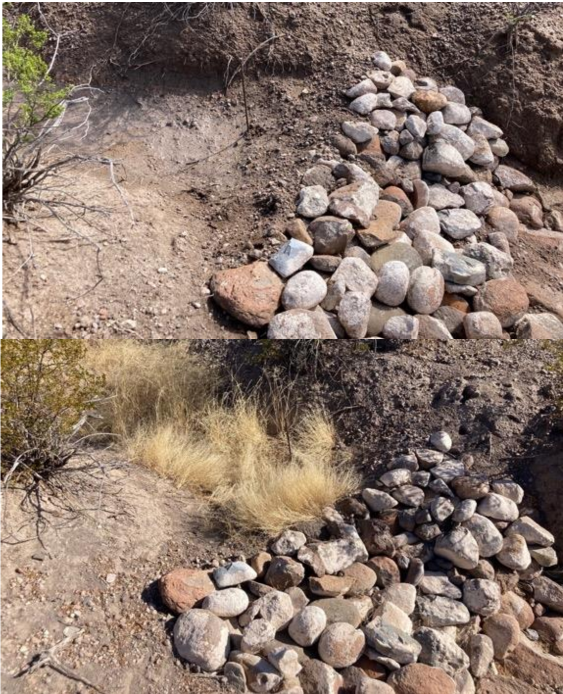
Figure 48. Photographs of a leaky rock structure built in April 2021 on the Alamito Creek Preserve.. The top photo shows the structure one month after construction and after a recent rain. In 2023, new plant growth on the upstream side of the structure can be seen (bottom photo) where water has been slowed and sediment has been dropped and collected. (These structures of examples of low-tech approaches to restoring eroded sites as they help slow water and capture sediment that would normally be carried away in runoff).
