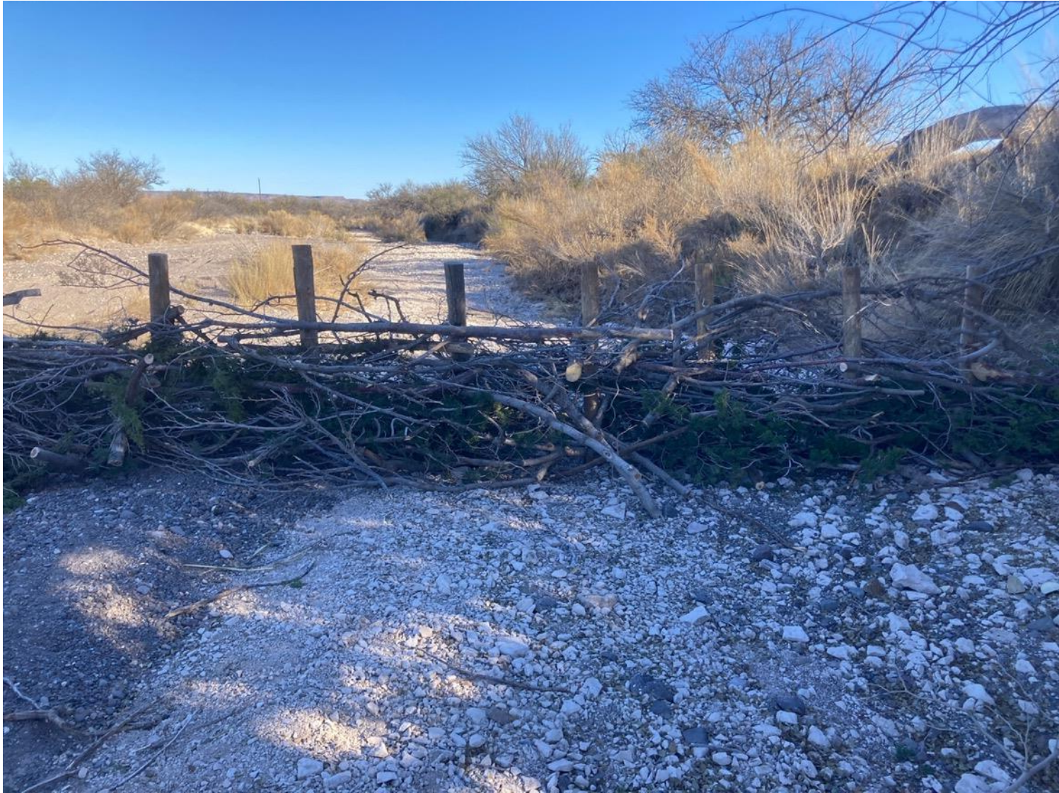
Figure 47. A completed brush weir structure composed of 6' pine posts woven with brush trimmings, in Matanoso Creek on Alamito Creek Preserve, December 2022. (Photo by Philip Boyd)
